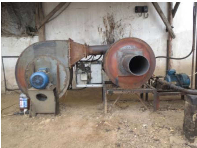
Figure 1 – Burner device for burning WOE
