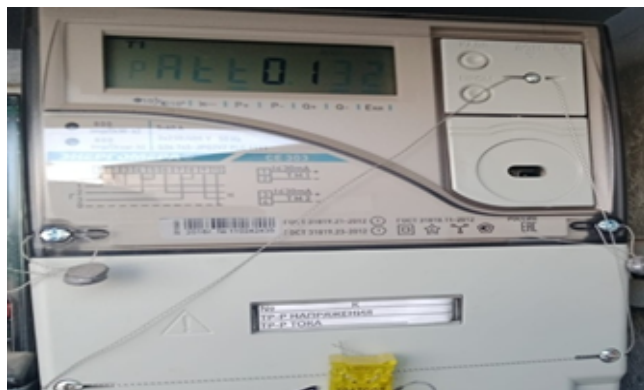
Figure 2 – Electric energy consumption metering devices Energy meter CE 303
