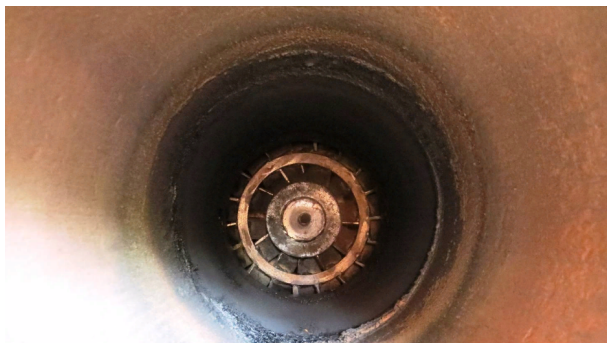
Figure 3 – Swirlers inside the combustion chamber
