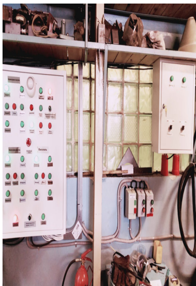
Figure 2 – Automatic control cabinet for hydraulic drive of the waste
